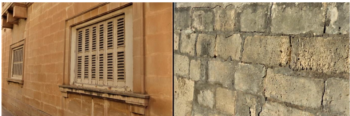
Comparative images showing Opuntia treated (left) and untreated walls (right)
